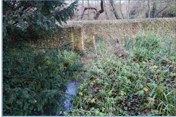
A flint wall used as a landowner boundary with a bricked archway for water to travel
